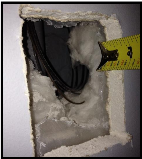
Figure 5.13: Hole in Interior Wall of SGH Office
