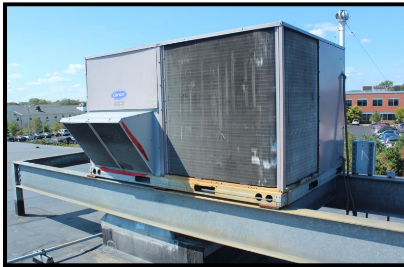
Figure 5.11: Packaged Rooftop Air Handling Unit on SGH Roof
