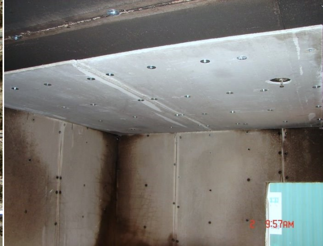
Figure 4-10: Additional construction of burn compartment walls and ceiling and deluge sprinkler head.
