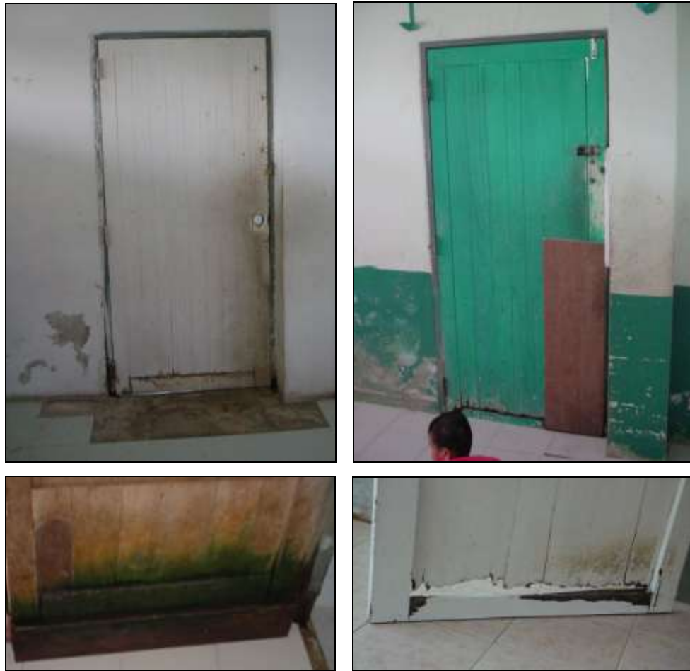
Figure 8: Series of Damaged Doors
