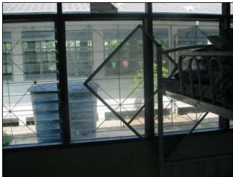
Figure 3: Damaged Window Screen
