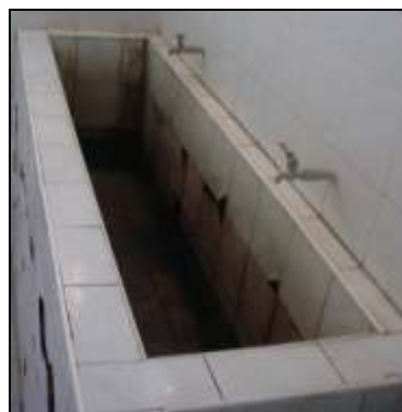
Figure 6: Trough with Cracked Tiles and Discoloration
