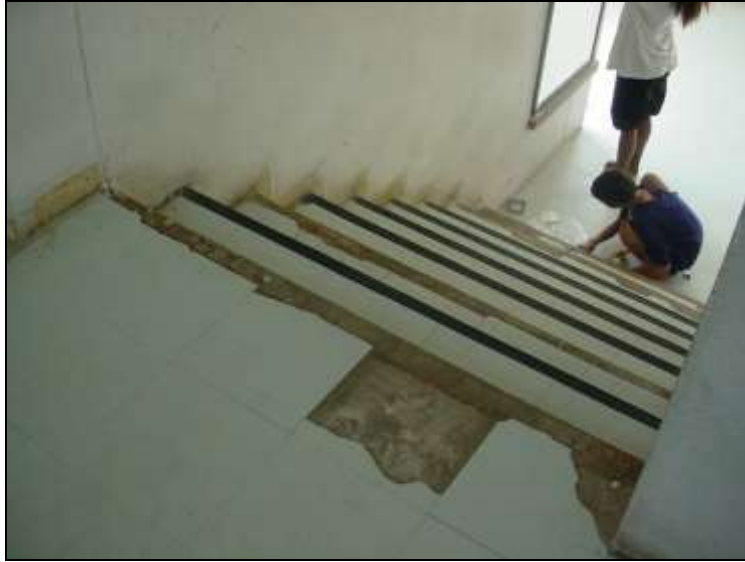
Figure 7: Cracked & Missing Tiles on Stairway
