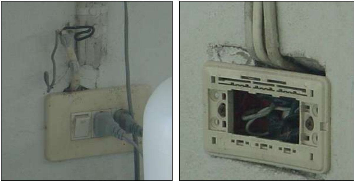
Figure 12: Example of Exposed Wires (Left) & Outlet without Cover (Right)
