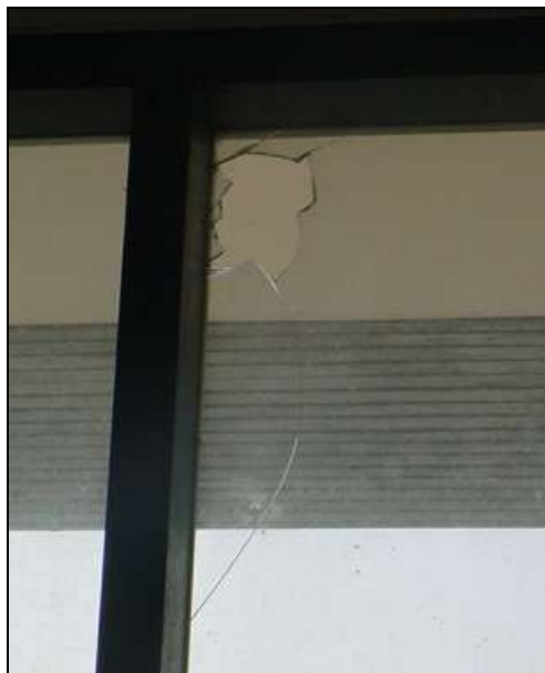
Figure 11: Example of Window with Broken Glass
