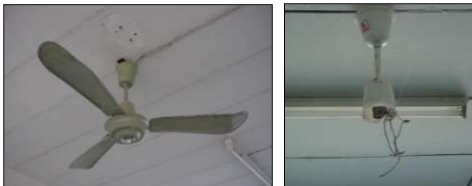
Figure 14: Metal Ceiling Fans without Cage (Left) and with Missing Blades (Right)
