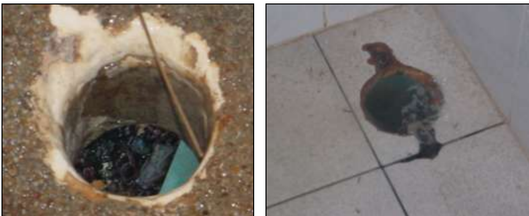
Figure 10: Examples of Coverless (Left) & Clogged (Right) Drains
