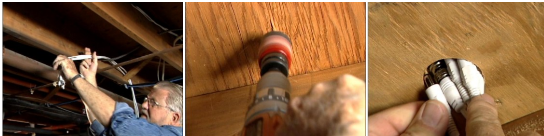
Cables are run through the basement and inserted into a room by creating a hole in the floor.
