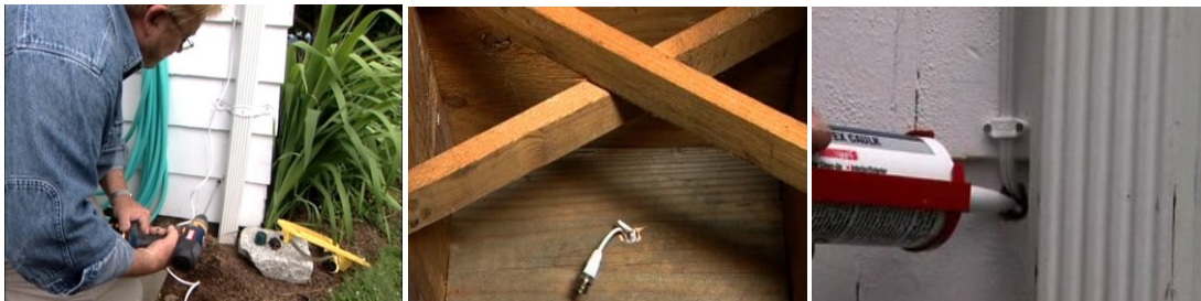
Power and video cords are inserted into the basement of the house by drilling hole through the house siding. The hole where the cords were inserted is then sealed.
