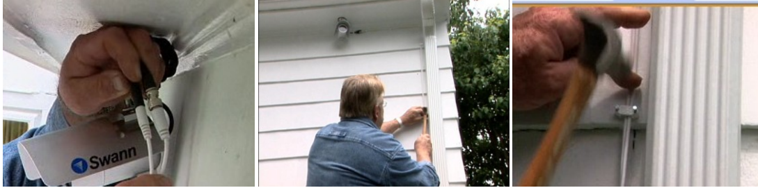
Camera is attached to mounting bracket, angled properly, and connected to power and video cables. Cable clamps are hammered into place to attach the power and video cords to the side of the house.
