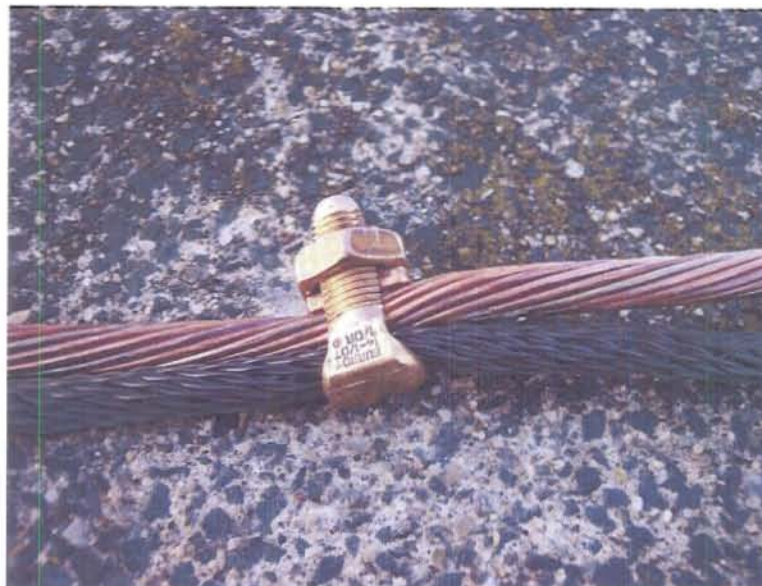
Figure 30: Lightning Protection Connection to Existing System
