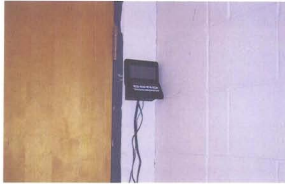
Figure 34: Weather Station Mounted in Closet
