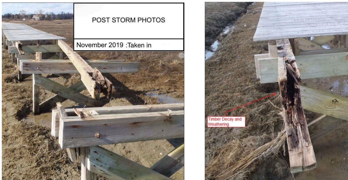
Figure 11: Shows the damage caused to Sandwich Boardwalk from 2018 Storm Surge.
