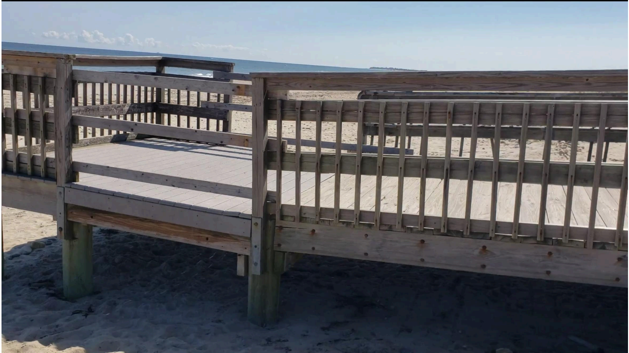
Figure 6: Image of the lower side of the Duxbury Parking Lot without ramp attached.
