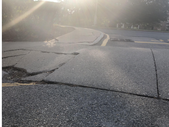
Figure 14-3: Some of the Rough Terrain PARV would Encounter on the Designed Pathway
