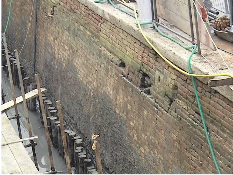
Figure 1: Example of canal wall damage
