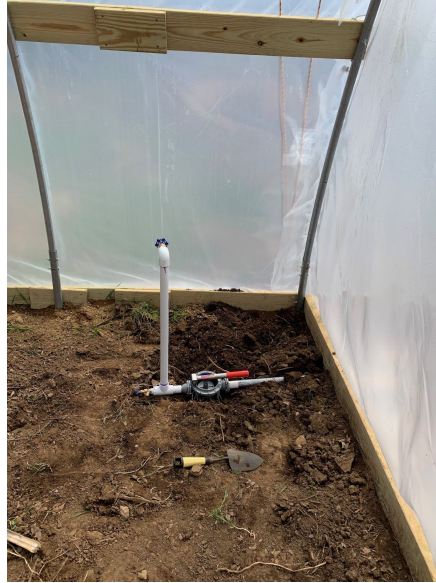
The water outlets inside of the greenhouse
