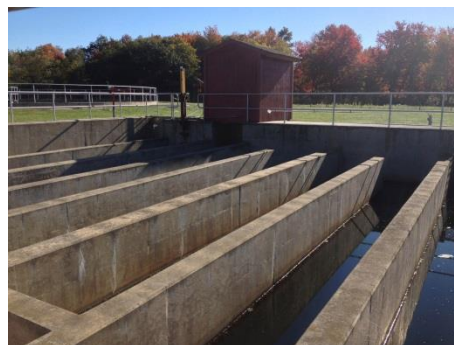
Figure 6: Chlorine Contact Chamber (Photo-credit: Mariel VanAtta, 2013)
