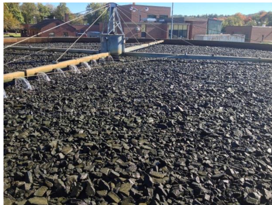
Figure 4: Gardner WWTF Trickling Filter (Photo-credit: Mariel VanAtta, 2013)
