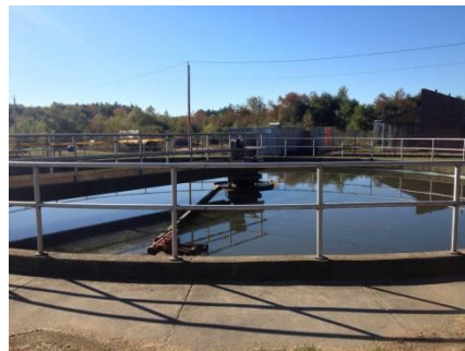
Figure 3: Gardner WWTF Primary Clarifier (Photo-credit: Mariel VanAtta, 2013)
