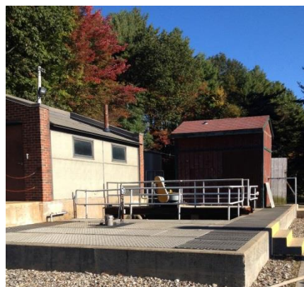
Figure 2: Gardner WWTF Headworks (Photo-credit: Mariel VanAtta, 2013)
