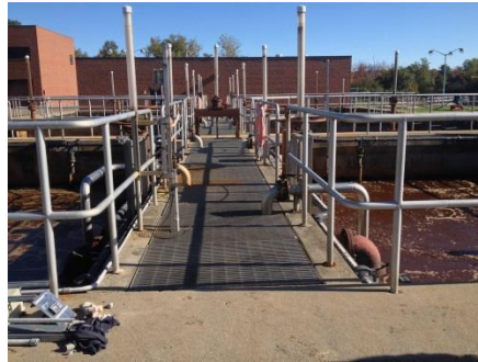
Figure 5: Gardner WWTF Activated Sludge Aeration Basins (Photo-credit: Mariel VanAtta, 2013)
