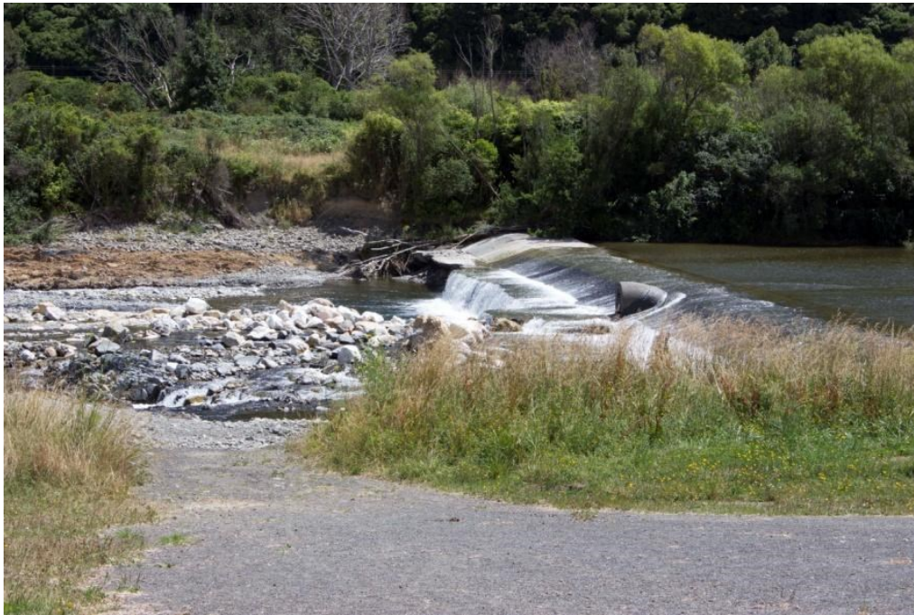
Figure 10: Erosion at Silverstream Sewage Pipe
