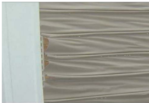
Figure 1. Vinyl Siding Distortion 5
