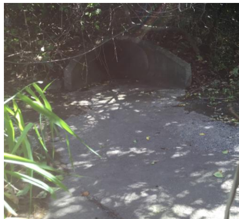
Figure 3: Discharge Pipe to Basin Weir
