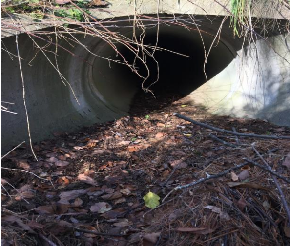
Figure 11: Dry Clean Water Bypass
