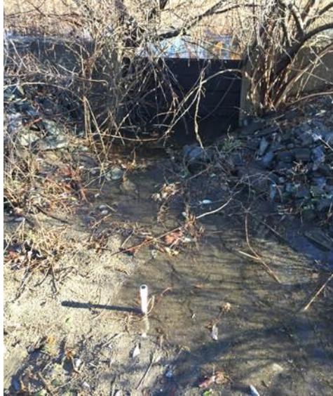
Figure 5: Pooling in Chamber 2
