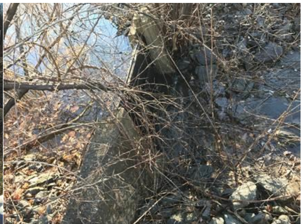
Figure 4: Weir between Chambers
