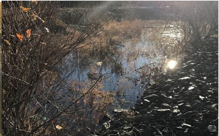
Figure 2: Pooling water in Chamber 1 (SouthWest View)
