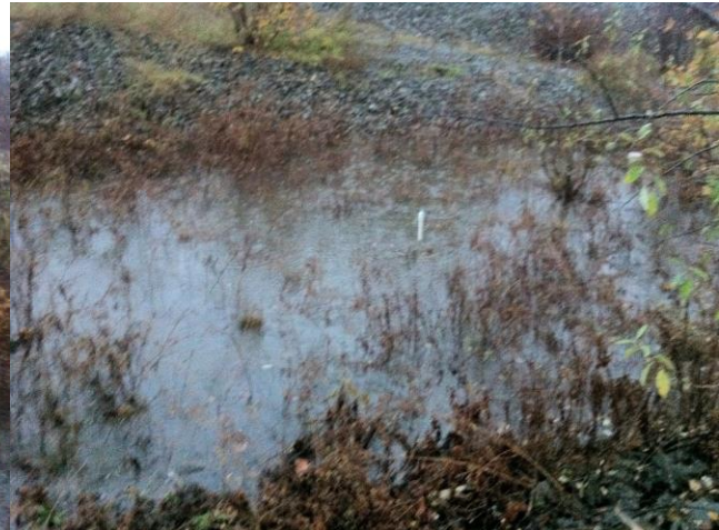
Figure 10: Chamber 1 with standing water
