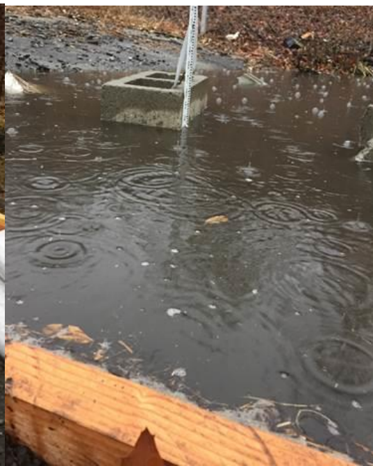
Photo 5: Seconds Before Overflow
