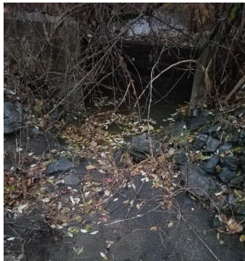
Figure 11: Chamber 2 with standing water at weir
