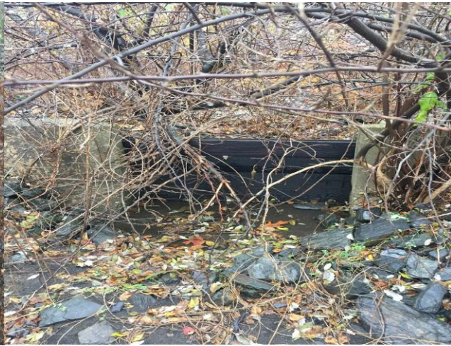
Figure 2: Pooling water in Chamber 2
