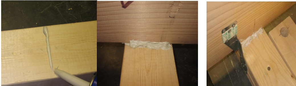
Figure 8: Liquid Nails being applied on bottom (left) and along edges (center) and Liquid Nails with hurricane strap (right)
