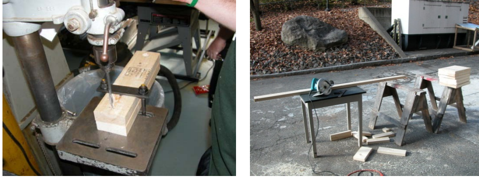
Figure 6: Drilling 1” holes in top plate section segment (left) and cutting 2 x 4 and 2 x 12 sections (right)
