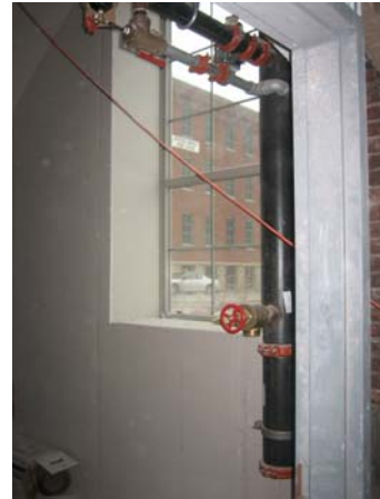
Figure 17: Standpipe in Stairwell
