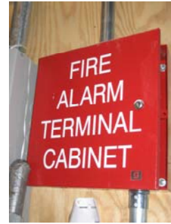
Figure 20: Fire Alarm Terminal Cabinet
