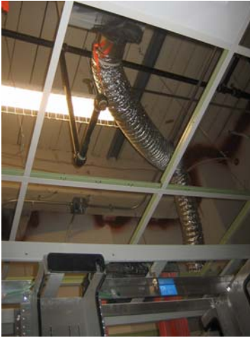
Figure 15: Sprinkler Head in Electrical Closet
