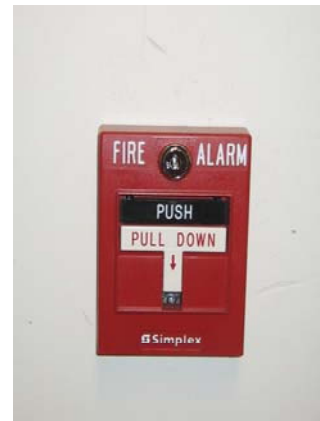
Figure 19: Manual Pull Station
