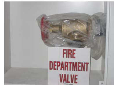
Figure 18: Fire Department Valve in Hallway
