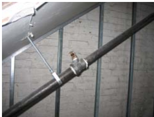
Figure 16: Upright Sprinkler Head in Stairwell
