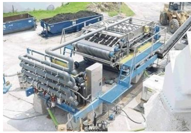
Figure 1: Dewatering Belt Filter Press
