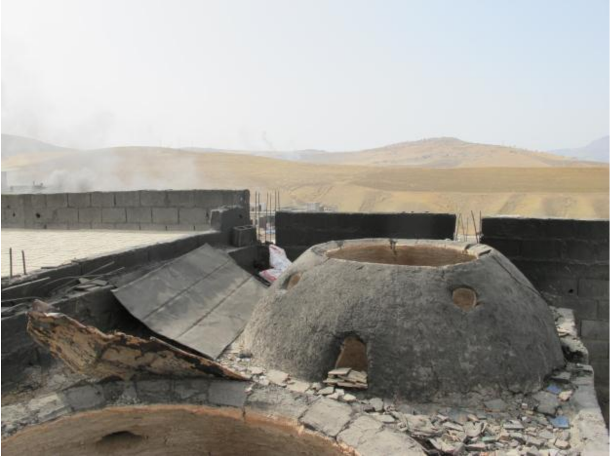
Figure 9: The top of the kiln as seen from the outside, roof level. Note the tiles drying in the sun to the left.
