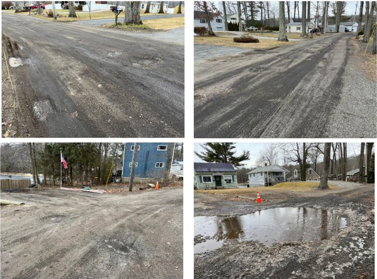
Figures 4.5 – 4.8: Pictures of road conditions at time of survey
