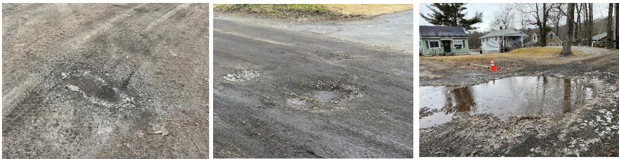
Figures 4.1 – 4.3: Potholes on Burncoat Ln classified as “Minor”, “Major”, and “Extreme” (left to right respectively)
