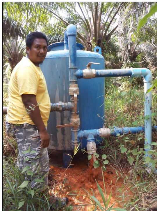
Figure 3: Existing iron treatment tank of well A4 in Baan Tha Thong Lang
