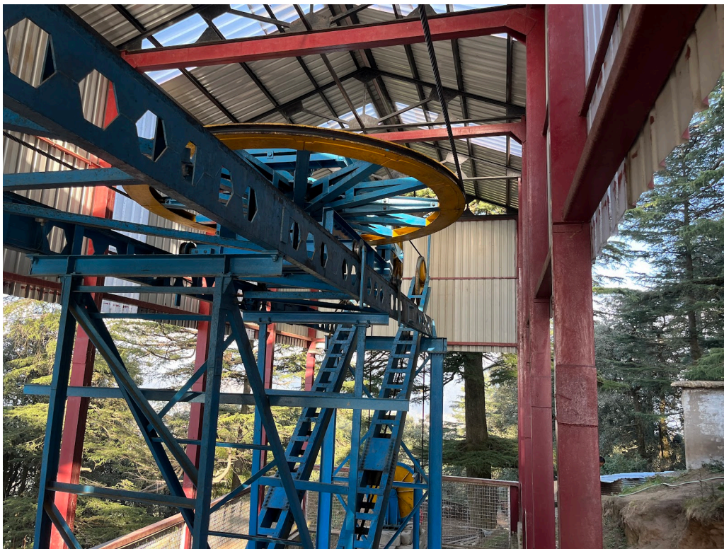
Figure 11: Mechanical system at top of Jakku Ropeway
