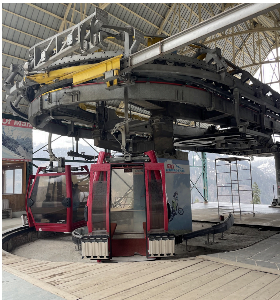
Top Station of Solang Valley Ropeway
