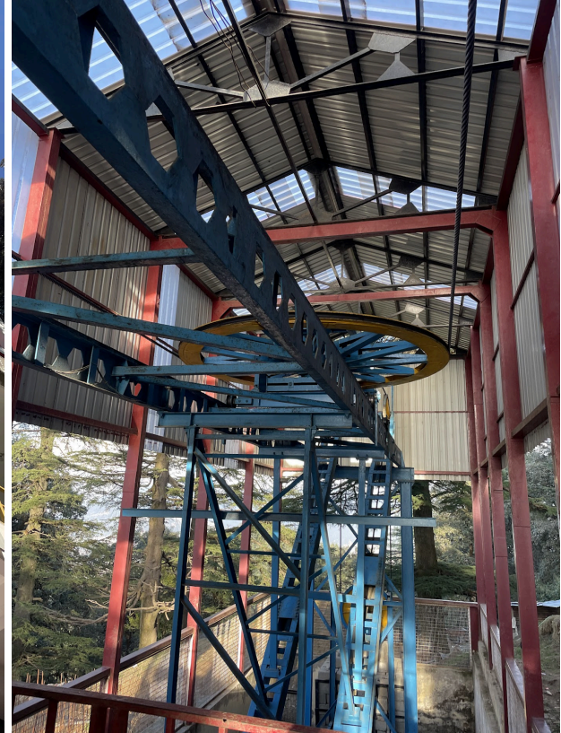
Mechanical system of Jakhu ropeway top station
