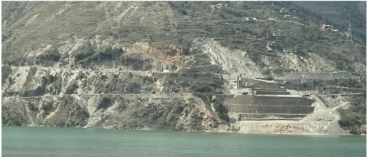
Figure 3: 2023 Pandoh landslide Damage to the future Kiratpur-Manali national highway and the shoring installed to fix the damage to stabilize the highway & the Baglamukhi Ropeway base station in Pandoh.
