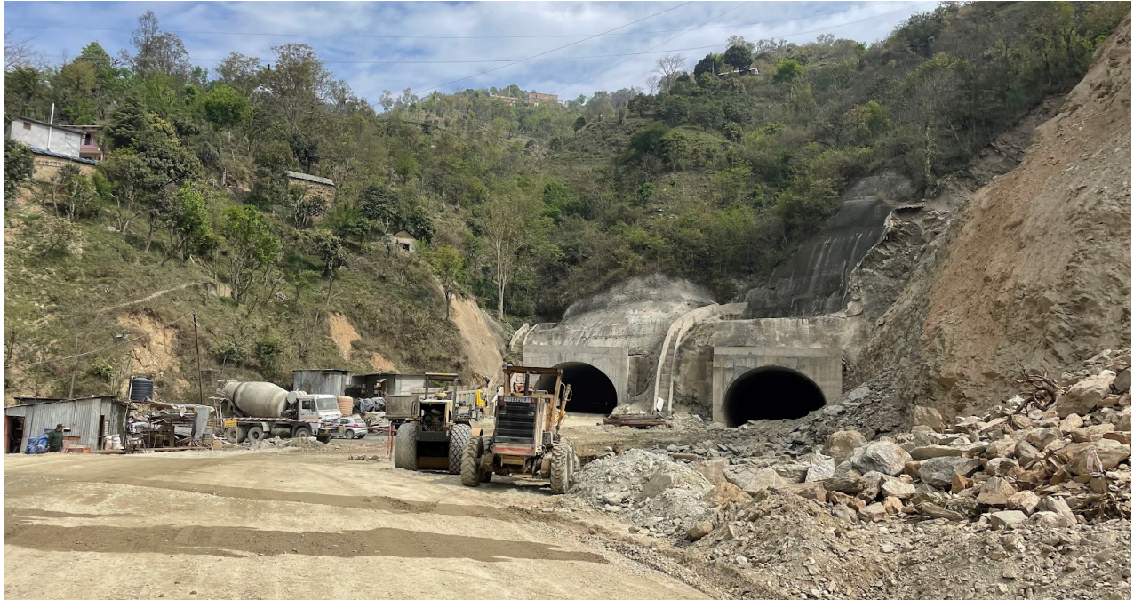
Figure 8: Construction on the tunnel for the Kiratpur-Manali national highway This will allow traffic to completely bypass Mandi town.
