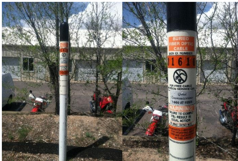
Figure 22: Buried Fiber Optic Cable Pole Right image shows pole close up
