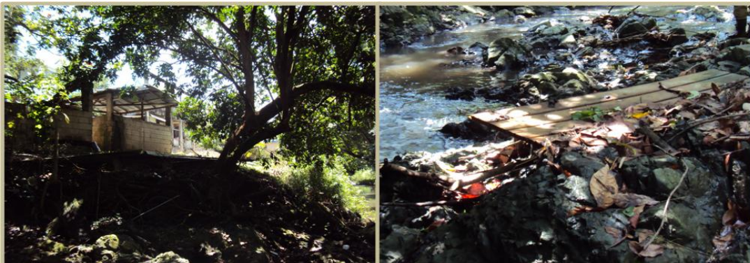
WPI-WP-38: (left to right): Dilapidated house and wooden plank
