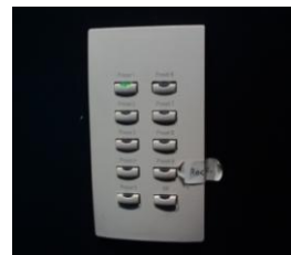
Figure 50: Control Panel in booth
