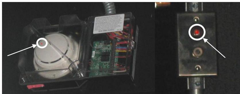
Figure : If either of these lights are solid red, this indicates an alarm has been tripped.
