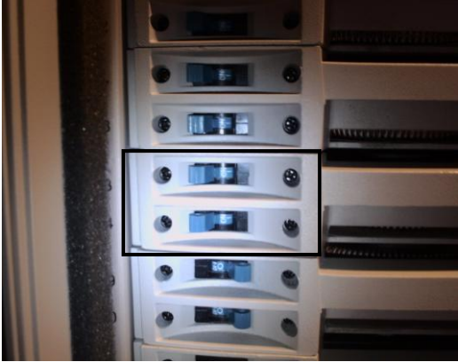
Figure 53: A dimmer card with the breakers engaged (Top, center). A dimmer card with the breakers unengaged (bottom)
