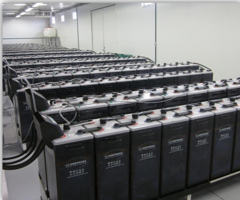
Figure 25: Solar-diesel battery banks
