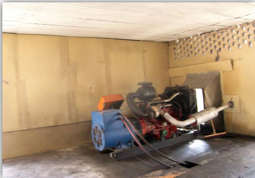
Figure 5: Original genset 2 (Hangula, [Photograph], 2011)
