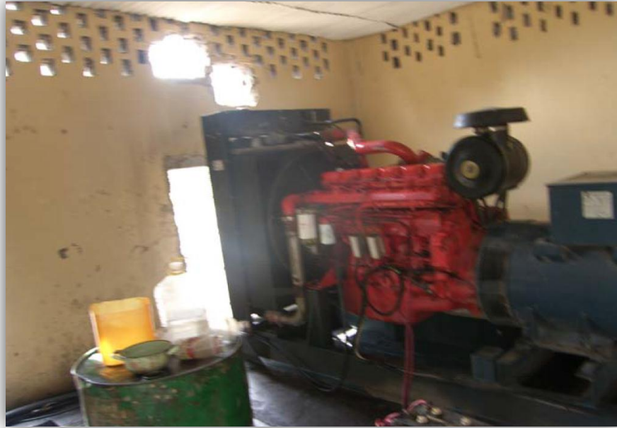
Figure 4: Original genset 1 (Hangula, [Photograph], 2011)
