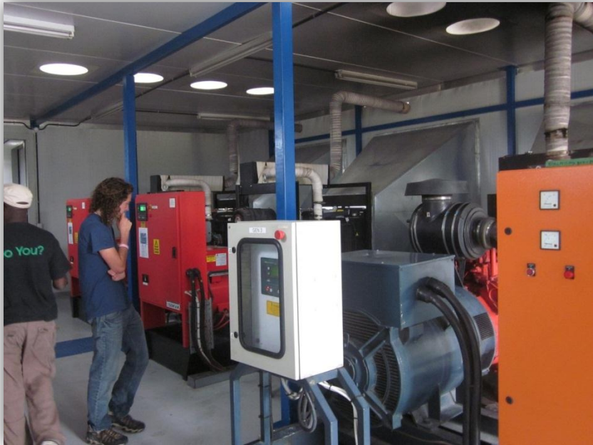
Figure 22: Diesel generator room of the solar-diesel hybrid system
