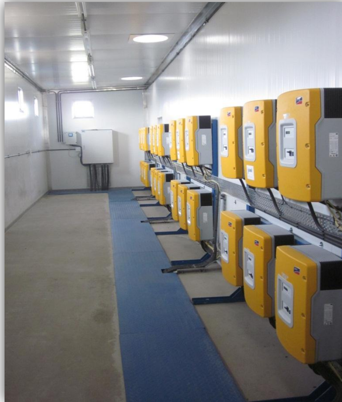
Figure 24: Solar-diesel hybrid system inverters
