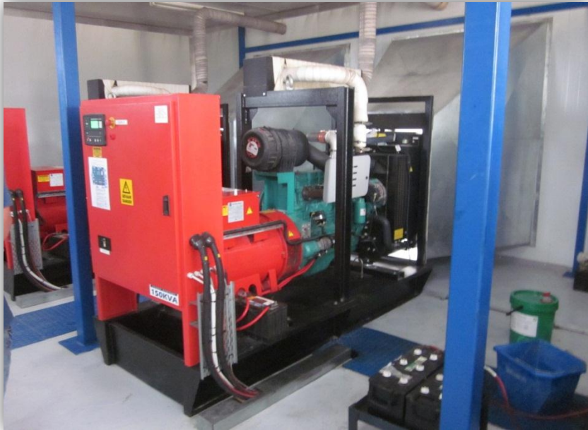
Figure 23: One of the 350 kV diesel generators
