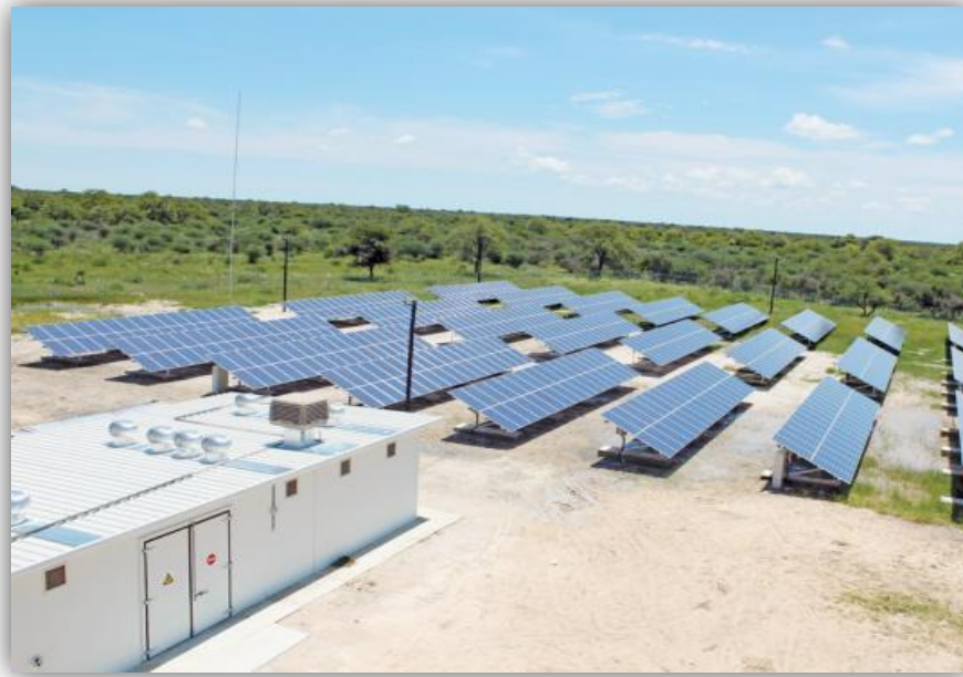
Figure 7: Solar diesel hybrid array—Tsumkwe, Namibia (DRFN, 2011)
