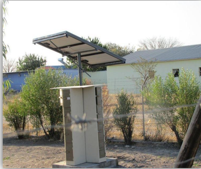
Figure 27: Solar kiosk installed in Tsumkwe Central at the Councilor's office (Hangula, [Photograph], 2011)
