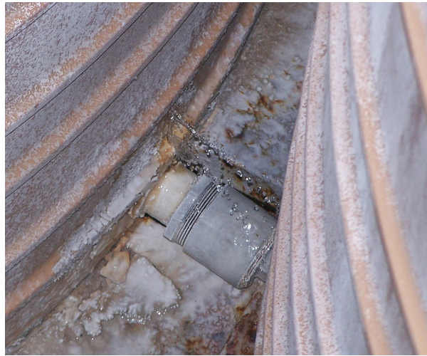
Figure 5.2: A leak in one of the NamWater storage tanks
