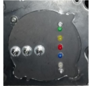
Figure B18: Panel Lights and Switches
