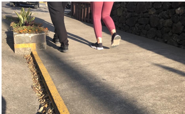
By adding a 2-3 inch space between the sidewalk and the road, maximum drainage to an underground culvert is achieved.
