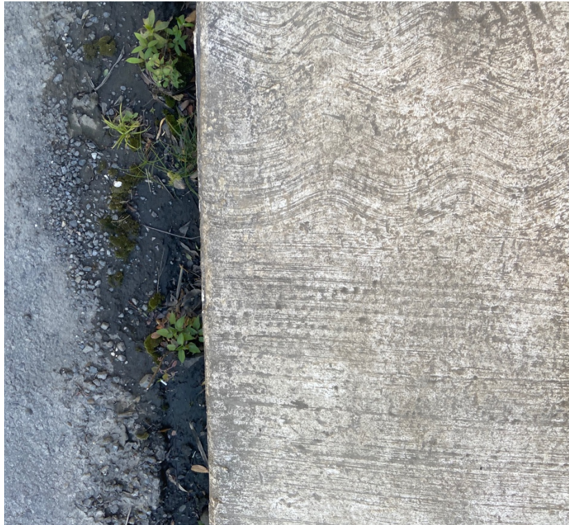
Figure 10: A non-slip surface on a sidewalk in Monteverde located between CASEM and Hotel Belmar.
