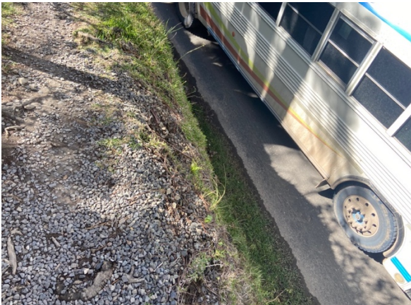
This sidewalk is elevated high off the ground; much higher than the bus in the picture for reference. A pedestrian could easily trip on the bigger rocks or roots in the sidewalk and fall off the ledge, possibly leading to injury.
