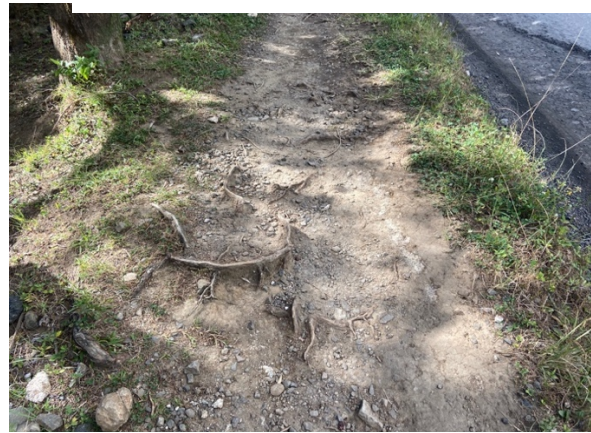
Large roots in the middle of this elevated sidewalk can cause tripping, and possible injury.
