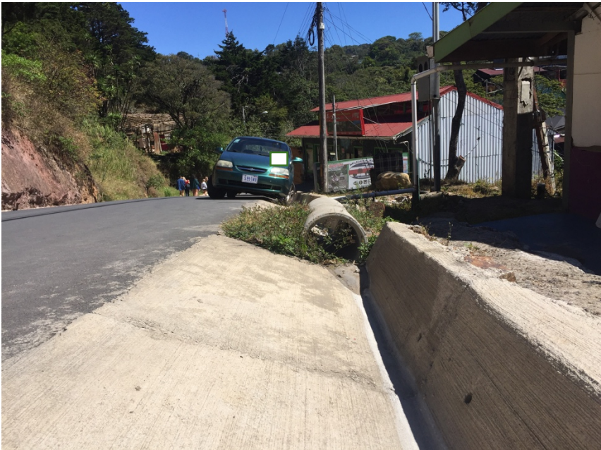
Sections of ditches are broken up by different types of drainage in many areas. This makes it more difficult to construct a continuous sidewalk.
