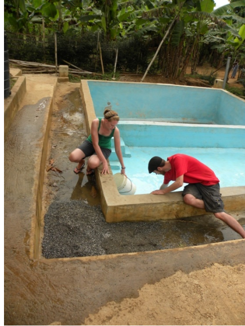
Figure 10. Collecting water for cleaning filter media
