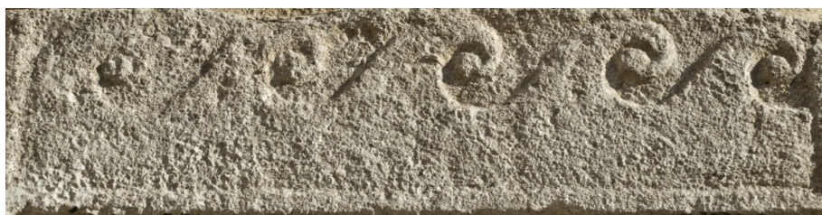
Figure 53: Exposure to the elements can wear down the hardest stone, rendering it illegible.
