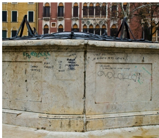
Figure 52: Wellheads, in public places and no longer actively used, are prime candidates for graffiti and abuse.
