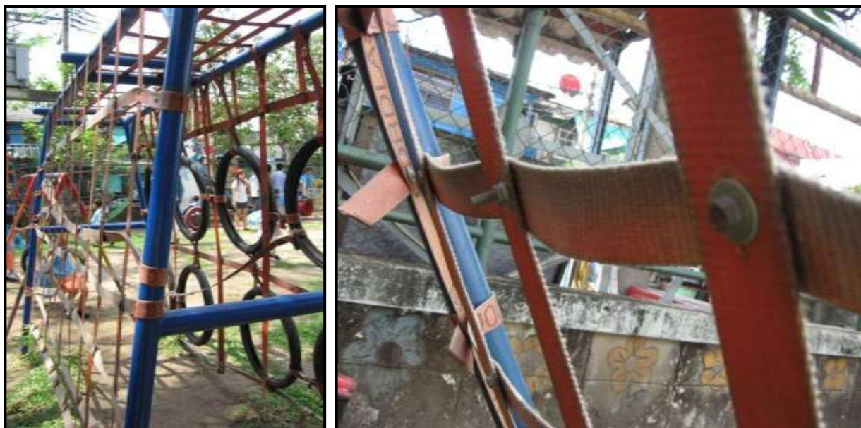
Figure 13. The tire strap climber has major safety concerns with missing bolts and broken straps (left), as does the cube climber with a protruding bolt on the underside of the climbing net (right).
