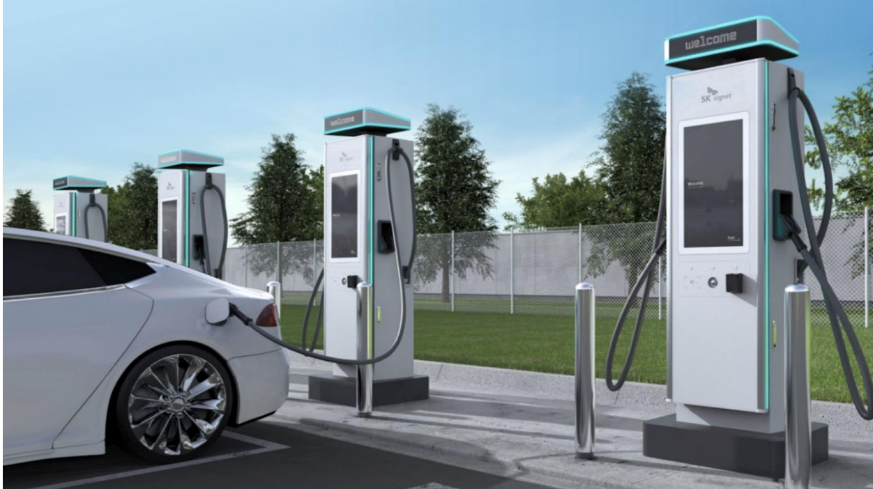
Figure 11: Standard Charging Station
