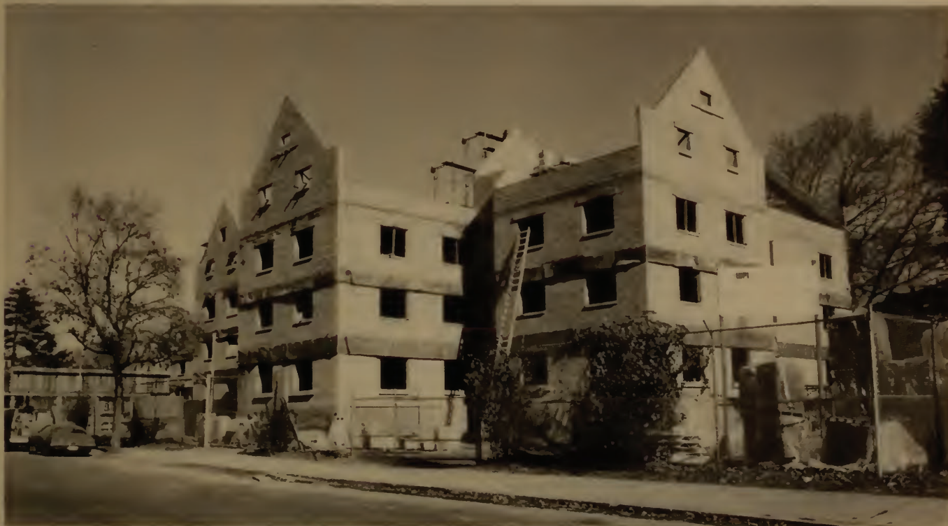
Unseasonably warm fall and early winter weather enabled easier construction of WPI's new residence center at the corner of Institute Road and Boynton Street. The new facility, to house and feed 229 students, should be open for September 1985 classes.
