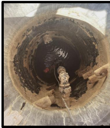
Figure 4.8: (Left) Flush Tank
