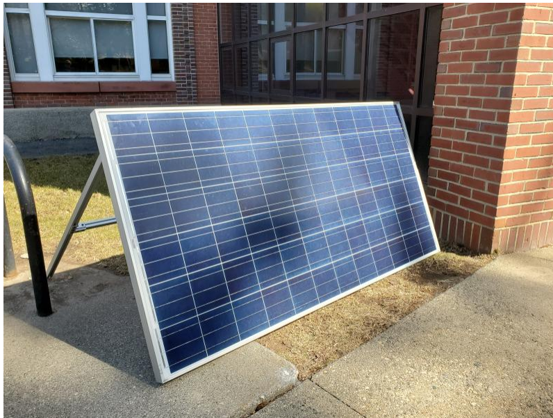
Figure 71: The solar panel is located to the left of the entrance to Atwater Kent Laboratories, next to the bicycle racks. This location was chosen for its proximity to the stairwell and the amount of sun available in that area.
