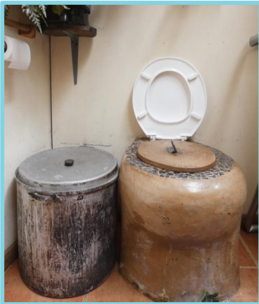
[Picture of a dry composting toilet]
