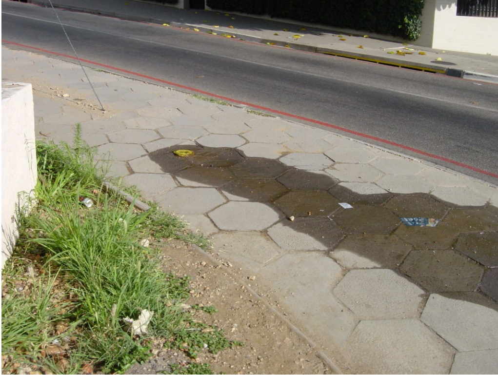
Figure 8. Leaking Water Main Shutoff Cap Near the Polytechnic of Namibia
