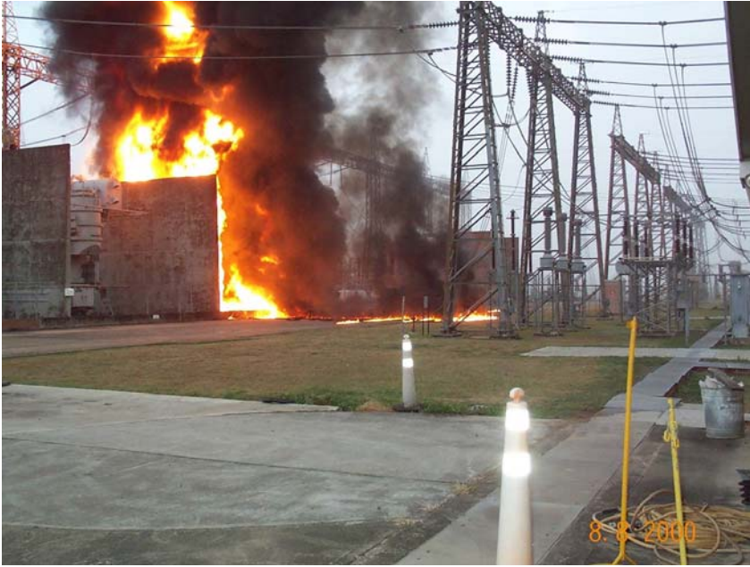
Figure 8.1 Typical Transformer oil fire (from FMGlobal).
