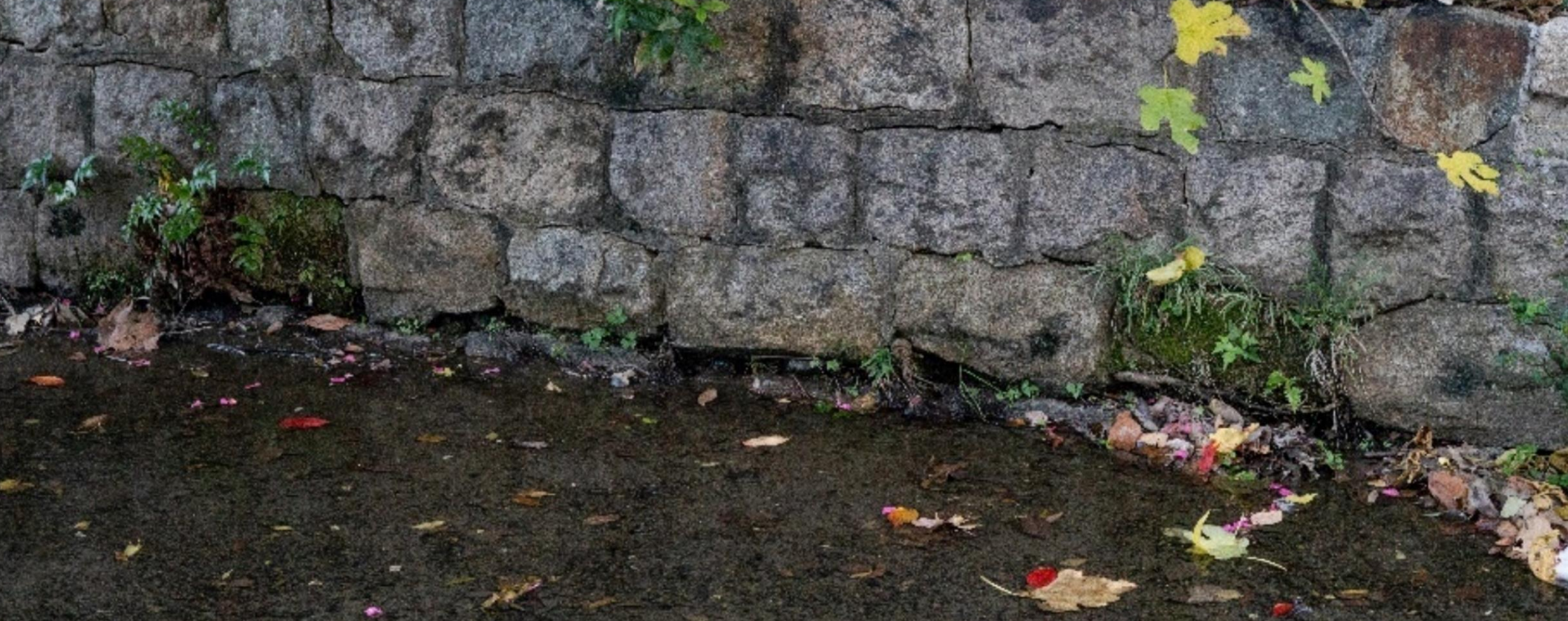
Figure 15: Example of Erosion Damage
