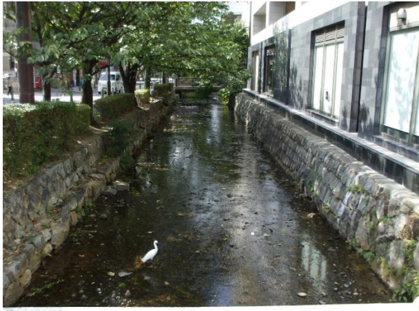
Figure 5: Oike-dori before repairs
