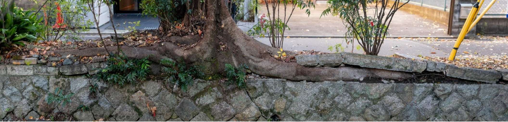
Figure 17: Example of Root Damage
