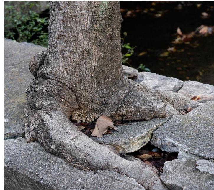
Figure 9: Example of root damage to the canal
