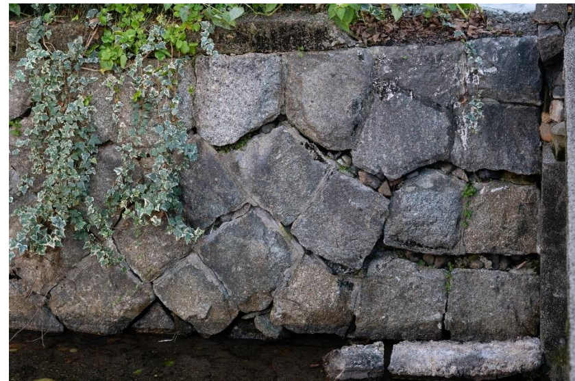
Figure 14: Example of Crack Damage
