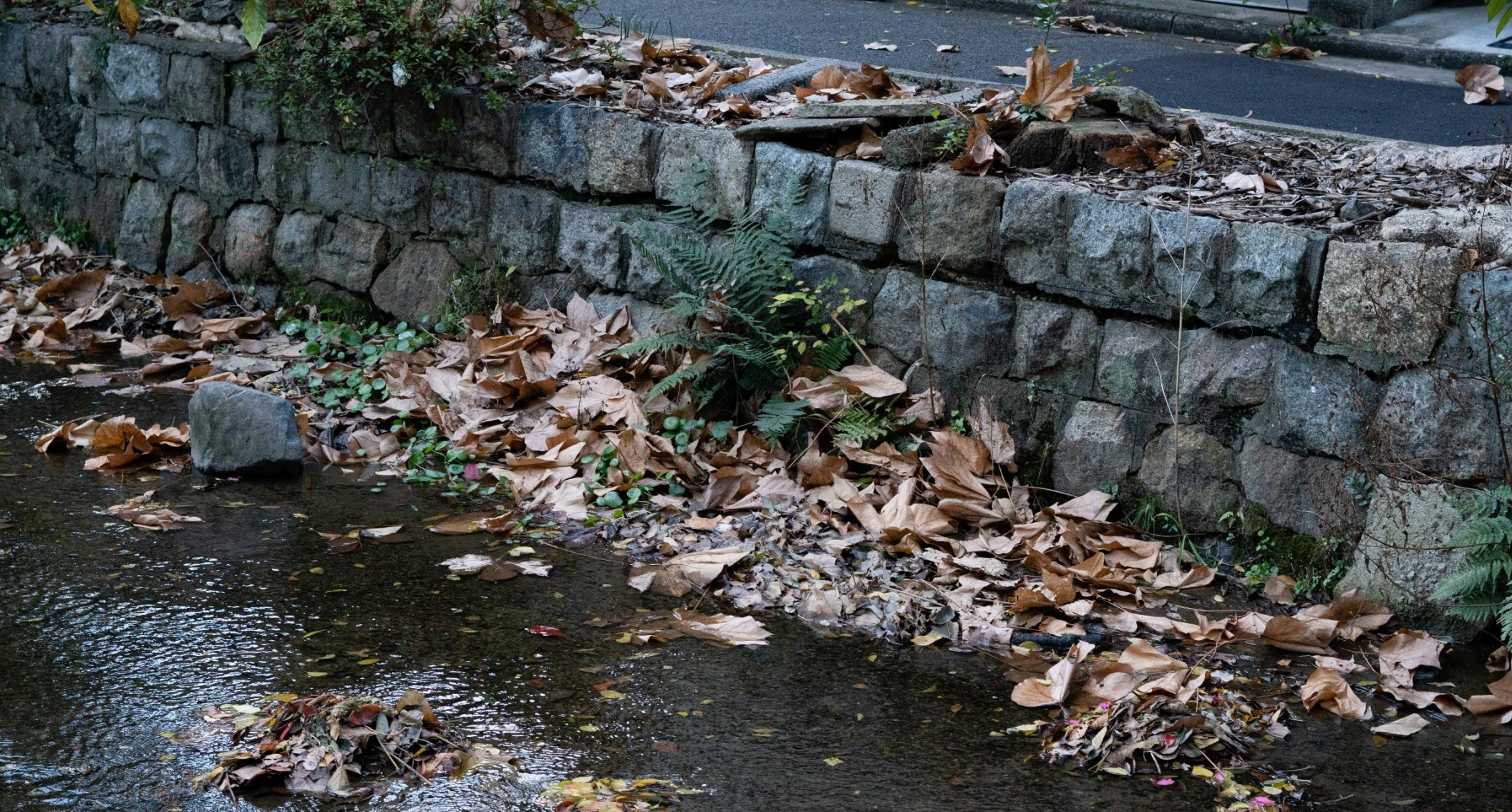
Figure 56: Leaves Piling Up Inside the Canal
