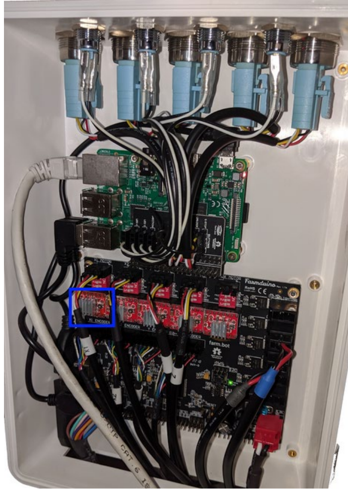
Figure 4.6 FarmBot electronics enclosure, damaged driver highlighted
