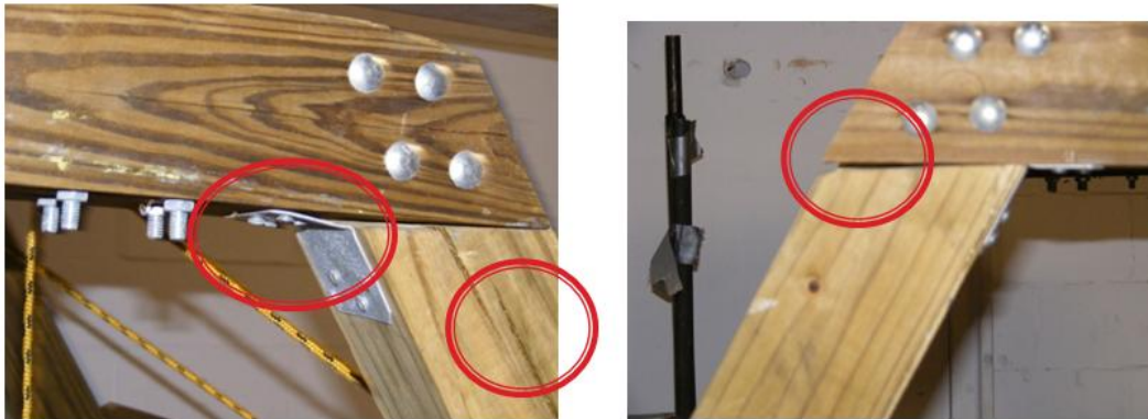
Figure 33 - Wear on A-frame
