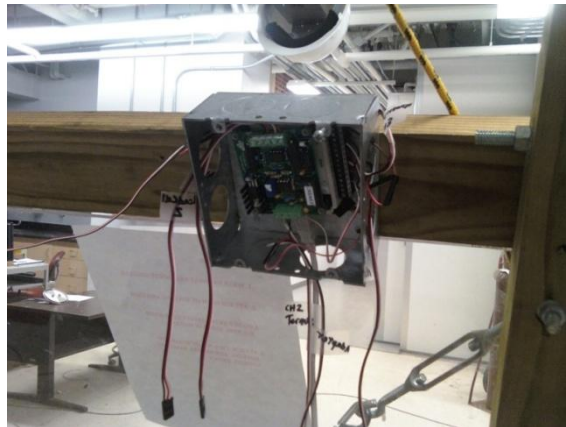
Figure 24 - Photo of Wiring setup of DAQ and instruments
