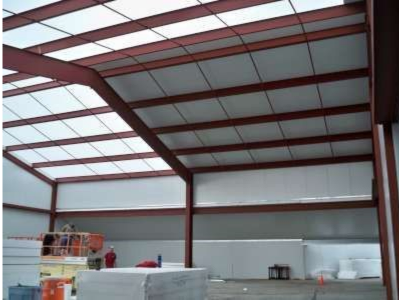
Figure 17: PermaTherm Roof Panels Being Used in Industrial Setting (PermaTherm, 2019)
