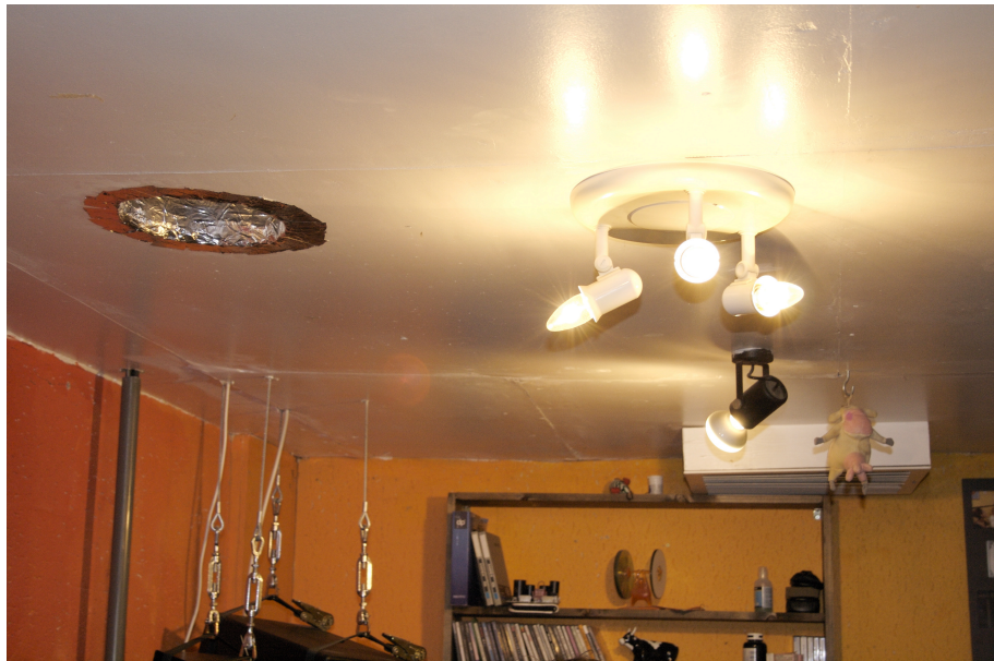
Photo 17: Base of Duct “Silencer” at Cowshed Studios
