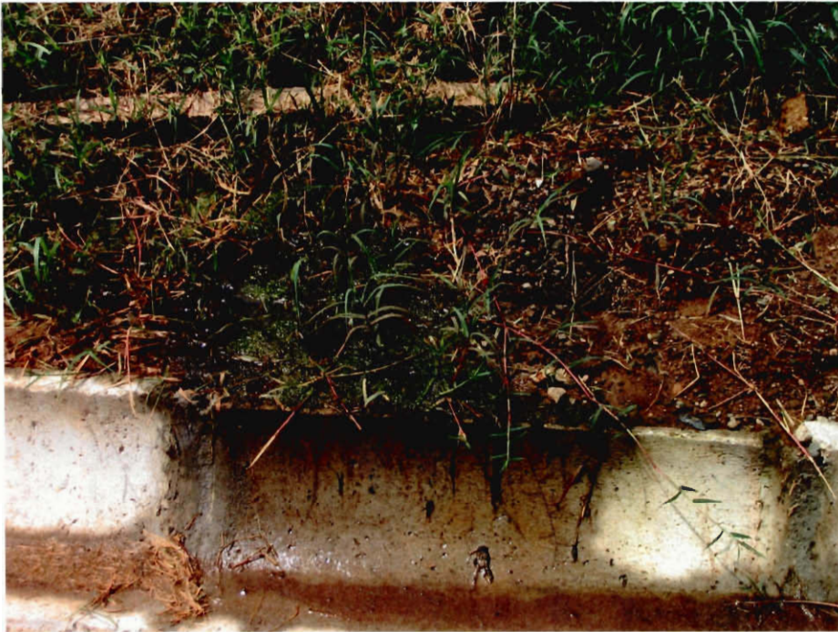
Figure 11: Area of landfill without an impermeable layer or leachate collection system. Note the green substance in the water. This is water that is highly contaminated and sits stagnant on the outside of a collection stream. The water will stay here until heavy rains wash it into the stream below.
