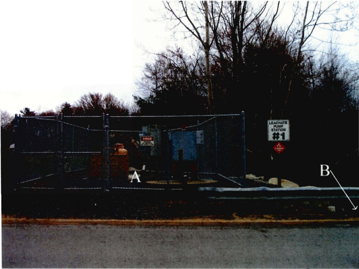
Figure 3. Leachate Pump Station #1
