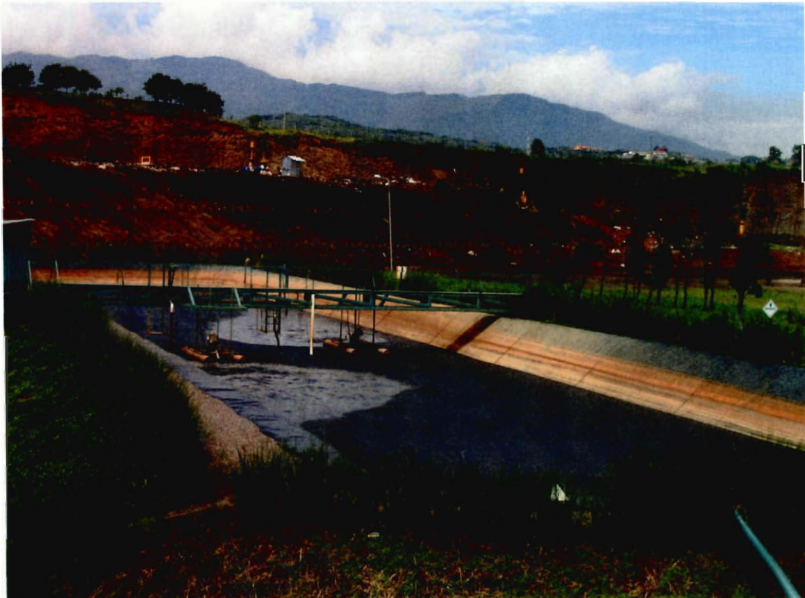
Figure 1. Water Treatment Lagoon
