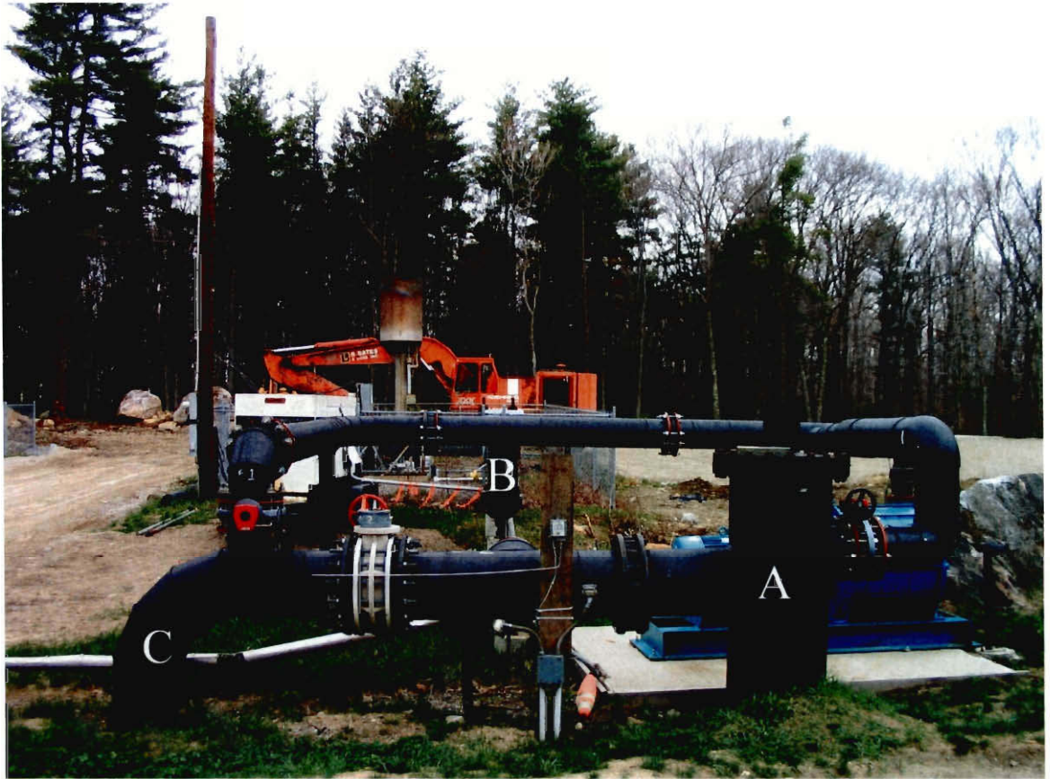
Figure 8. Collection and Transport Pipes
