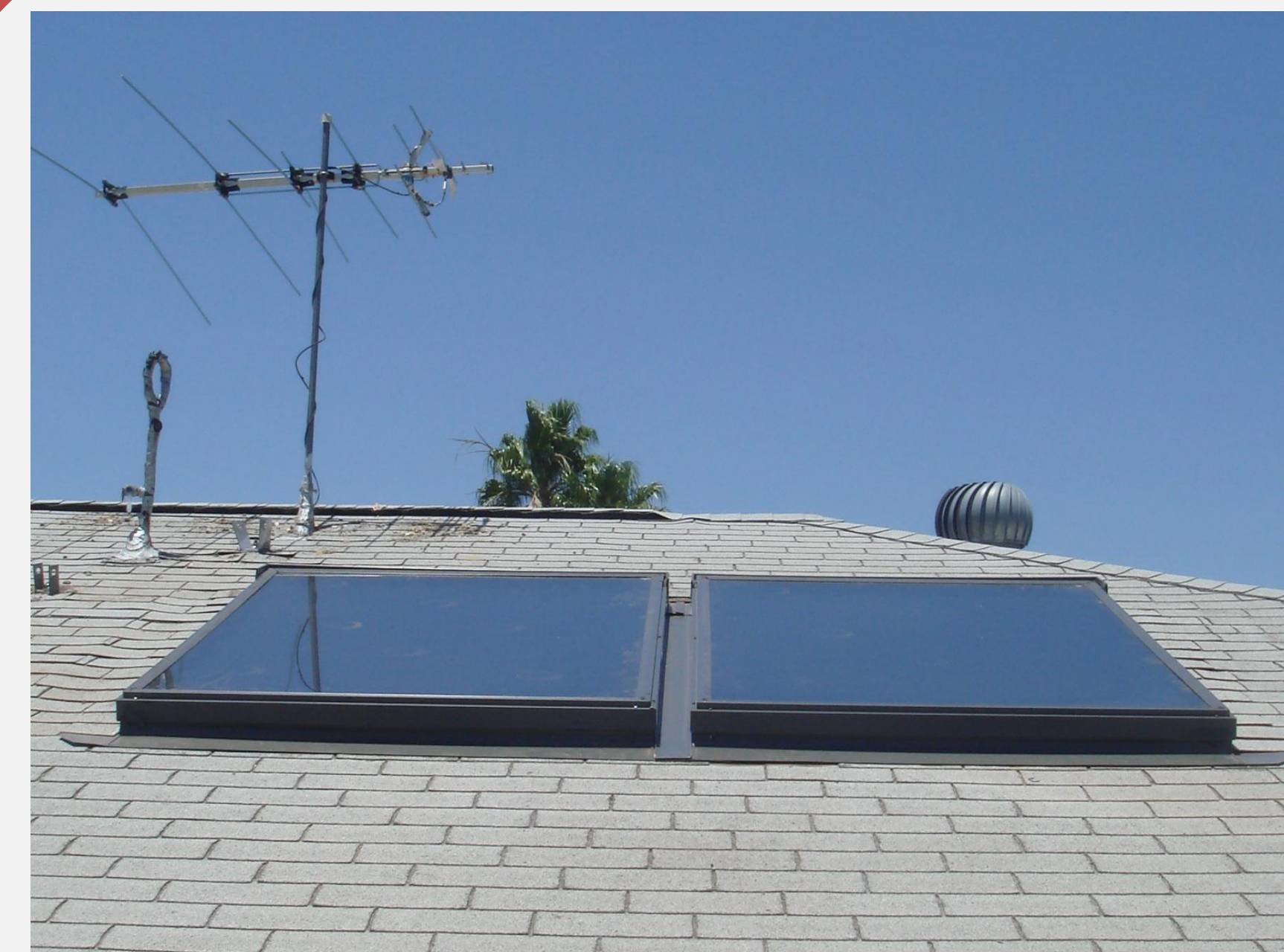
Solar water heaters on the roof converts sunlight to heat, reducing water heating bills from 50%-80%.
