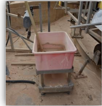
Figure 15: Secondary drainage bin
