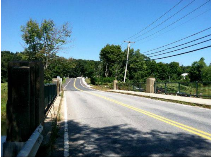
Figure 2: Dip Between Existing Bridge and CSX Bridge
