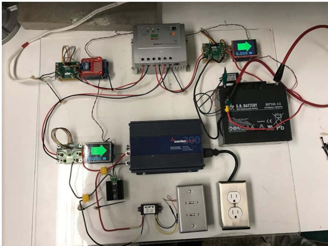
Figure 23. Solar Charging Station with Xbee Module
