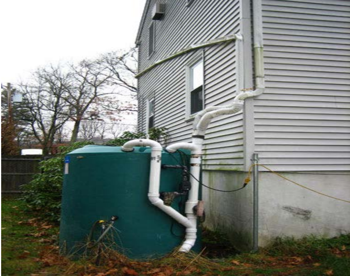
Figure 8: an 800 gallon rainwater harvesting system
