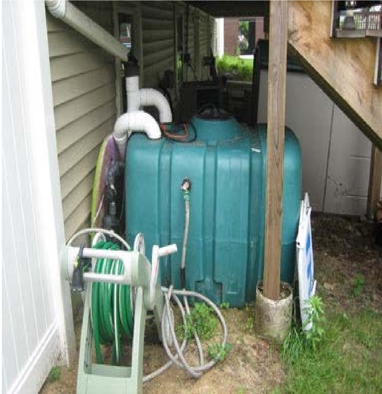
Figure 7: Example of a rainwater harvesting system used in one of the homes in Wilmington
