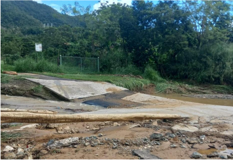
Figure A: Damages to a road in Las Carolinas after Hurricane Maria
