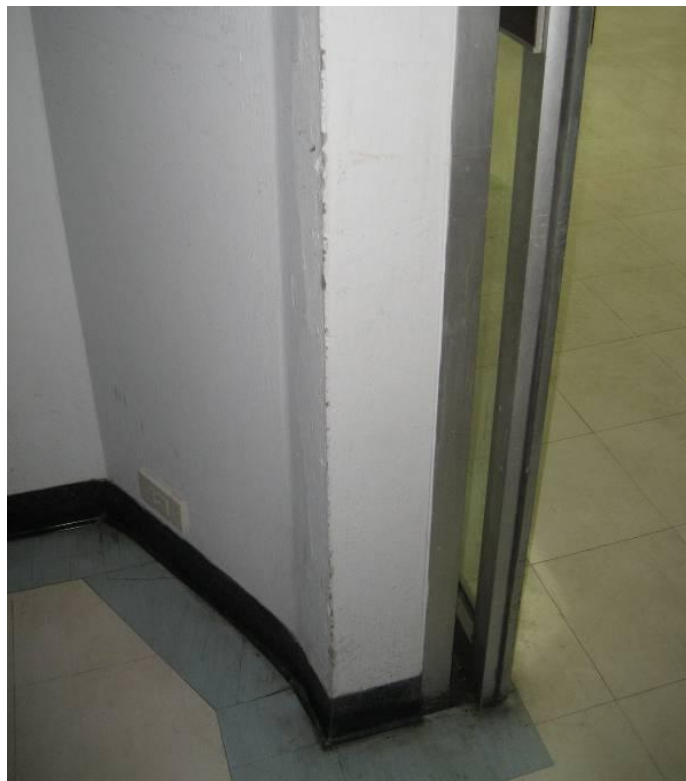
Figure 19: Damage of the Centre's Walls
